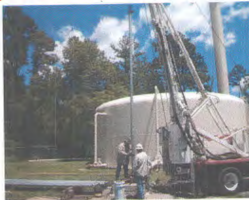
The installation of the new piping at the District's Well Water Pump #1.
